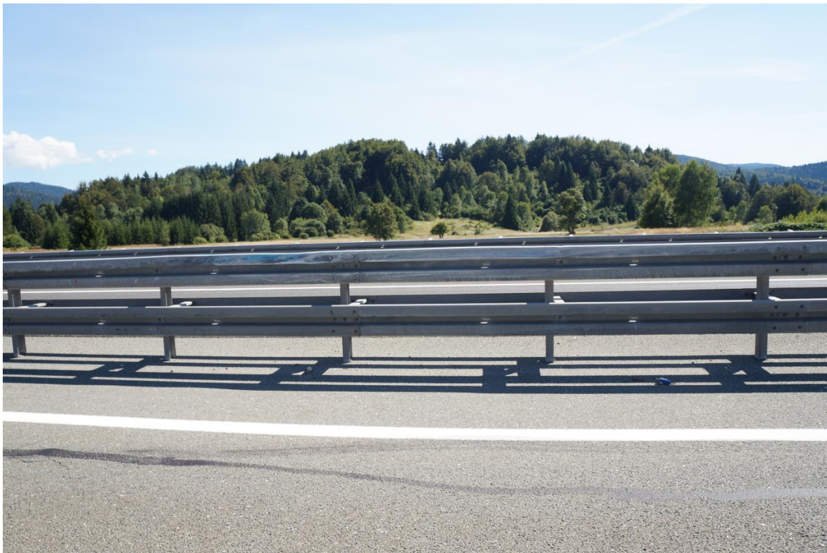
Picture 3 – Damage to the motorway guardrail
