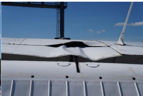
Picture 2 – Damage of the wing skin
