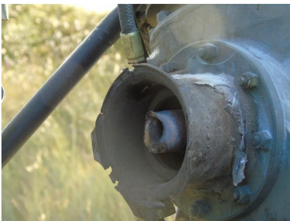
Figure 25 – Opening on the main gearbox
