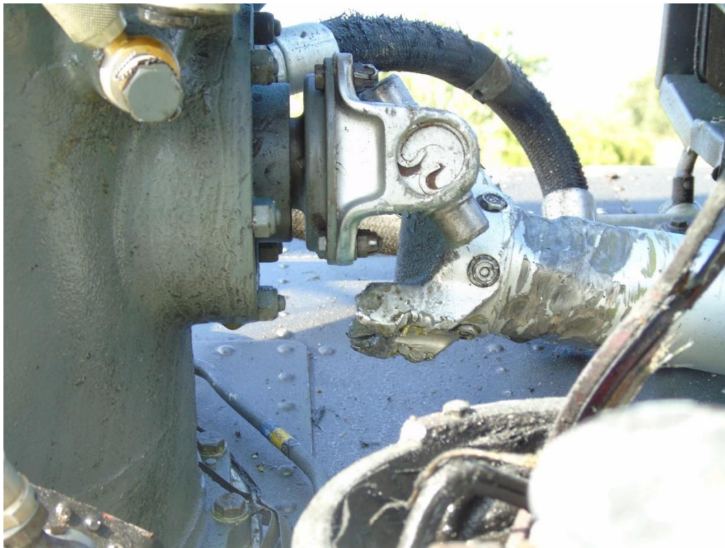
Figure 18 –Cardan shaft drive assy. at the cracking point
