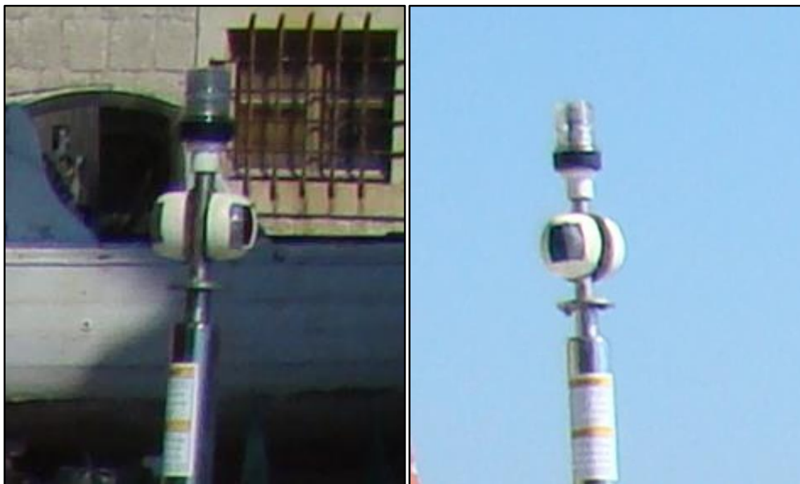
Picture 11 Showing of modifications by duct tape on the navigation lights
