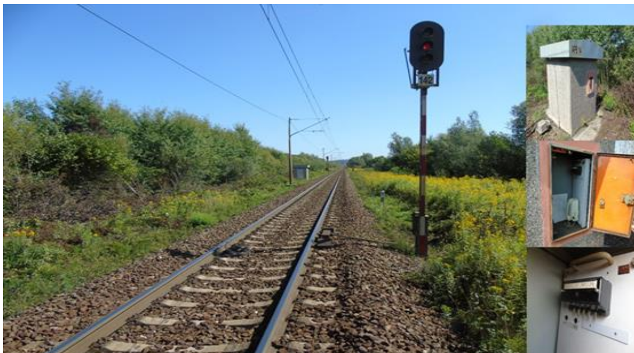
Figure 12. APB box with telephone (Image source: AIN)
