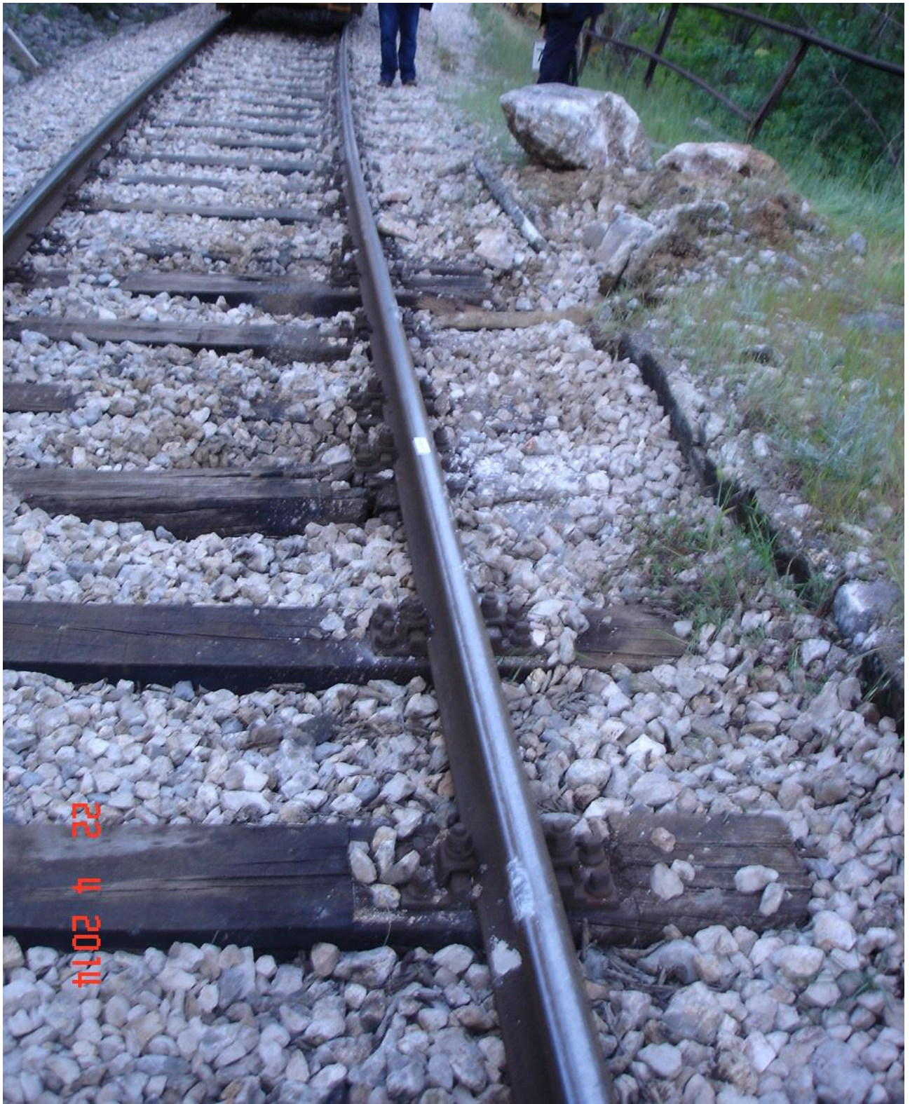
Image 4—Line damage at the point of the rockfall (image source: HŽ Infrastruktura d.o.o.)
